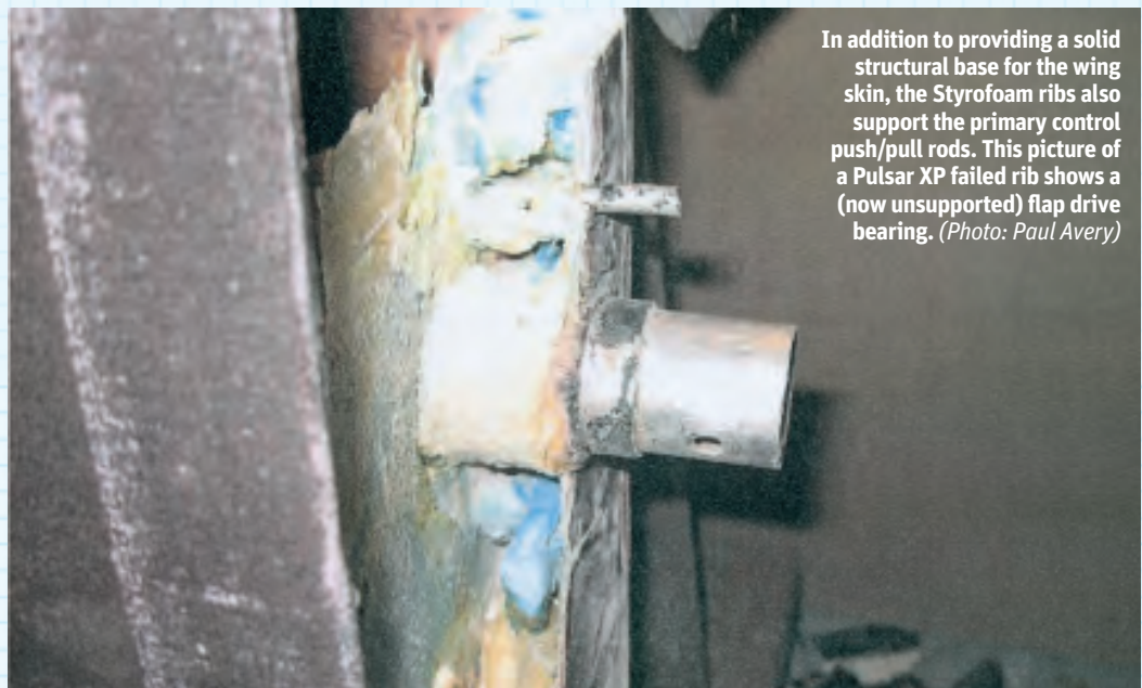
This is the sight that confronted Paul when he opened up the end rib on a Pulsar XP he is rebuilding. It looks like fuel vapour has encroached into the aft section of the wing from the leading-edge fuel tank vent. This is an early Pulsar XP and the Styrofoam ribs are covered with 1/16in plywood skin which, in turn, is covered with 6oz glasscloth. The foam ribs, while not particularly strong in themselves, are essential in distributing loads around the wing through to the main and rear spars. (Photo: Paul Avery)
