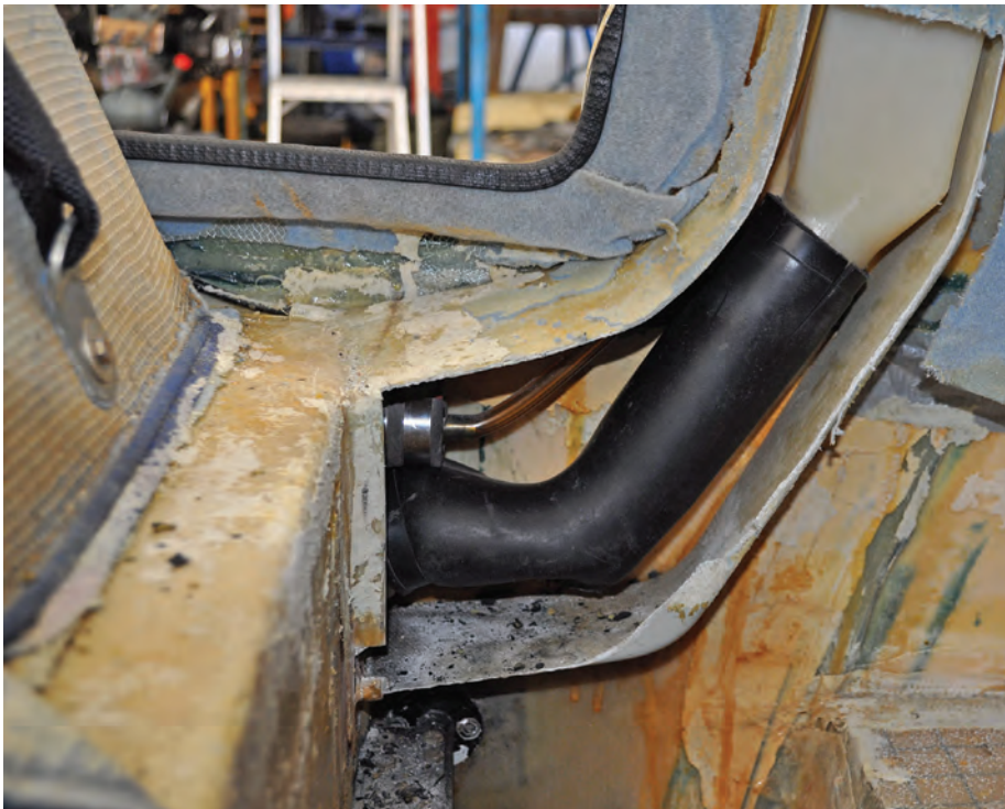
(Above) We showed this picture of a failed fuel inlet pipe in the December 2017 edition of Safety Spot and, as you may recall, the failure of this pipe has prompted the issue of an Airworthiness Information Leaflet , requiring checks on all Europa aircraft. (Photo: Malcolm McBride)
