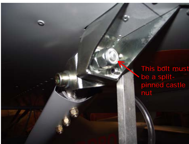
Fig 2. The wing strut to wing connection; an LAA Initial Acceptance Requirement (IAR-372-020) requires that the upper and lower wing strut fixings have their nyloc nuts replaced with castle nuts.
