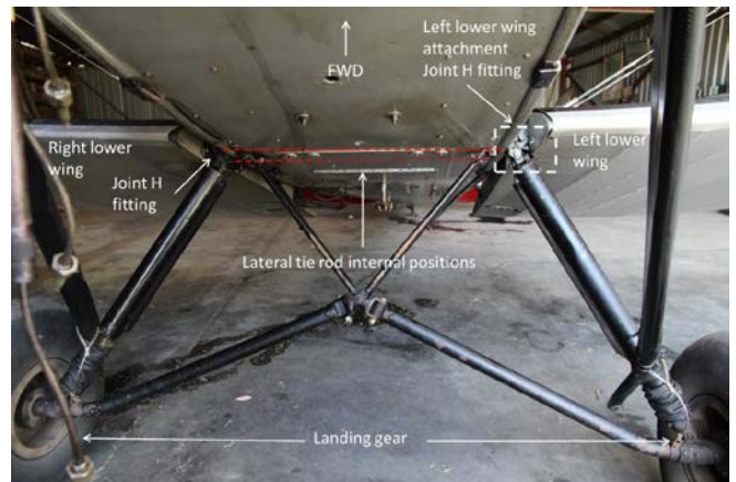
Fig. 1. View looking aft, showing the area of concern and position of Tie Rod.
