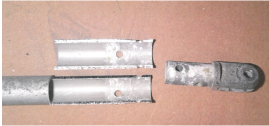
Fig. 1 A picture supplied by Murphy Aircraft showing the extent of the corrosion found in a recent inspection.
